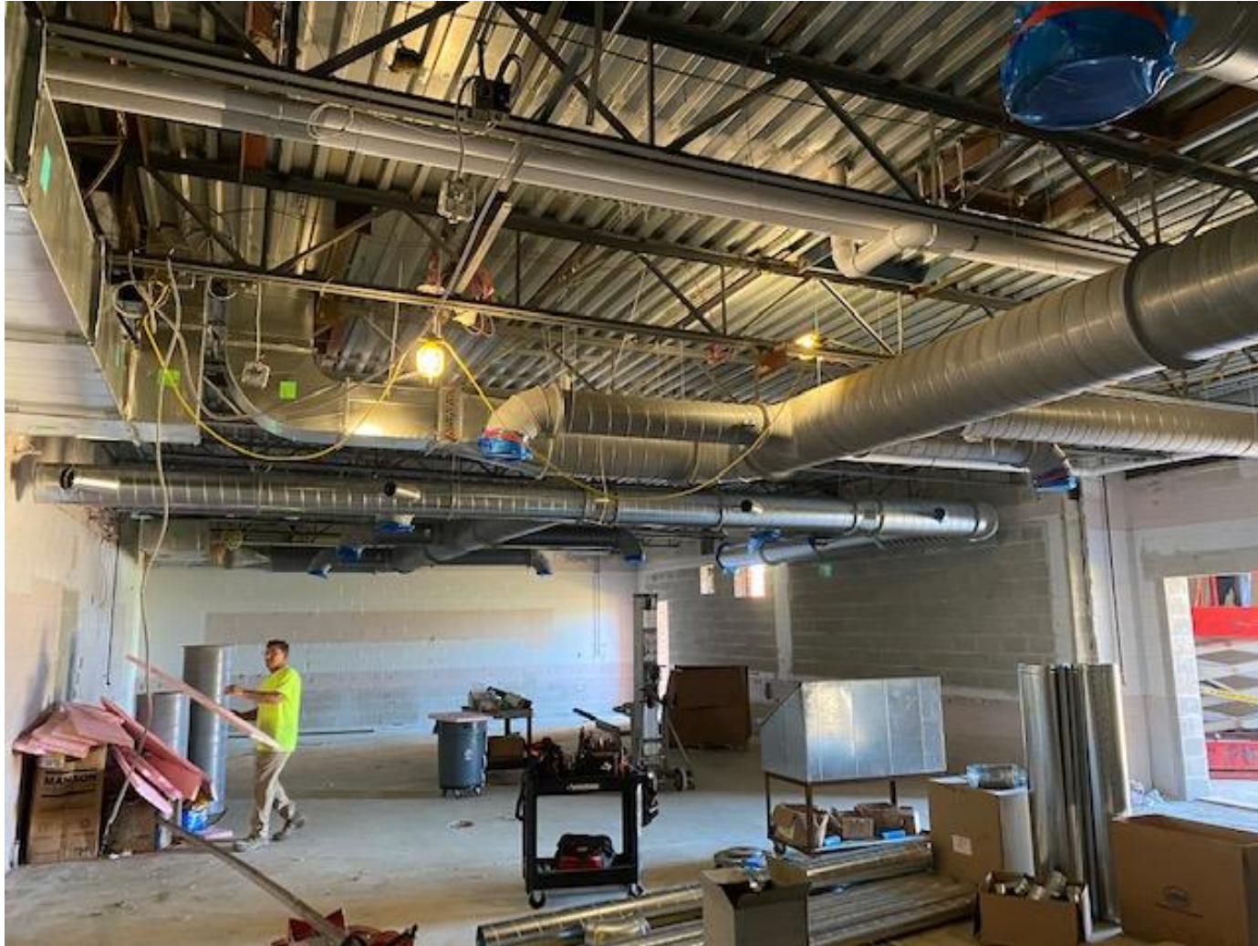
Ductwork In New Wood Shop (800 Wing)
