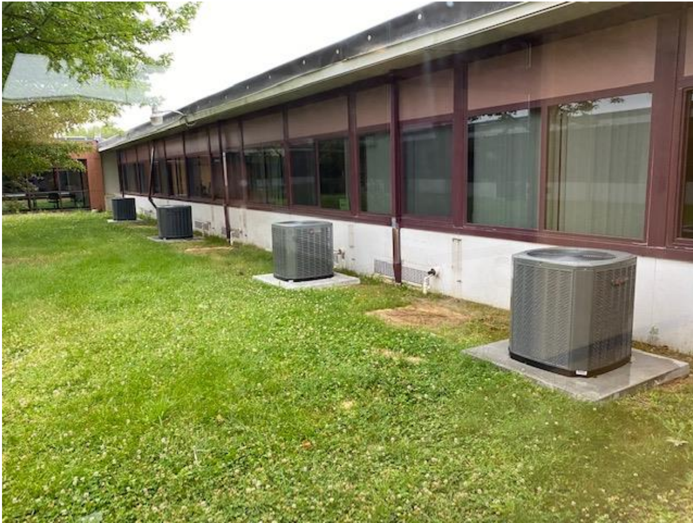
Condensing Units for Unit Ventilators at 400 Wing
